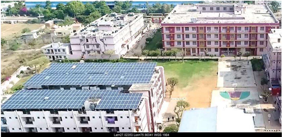
Solar Power Plant Installed at Roof
